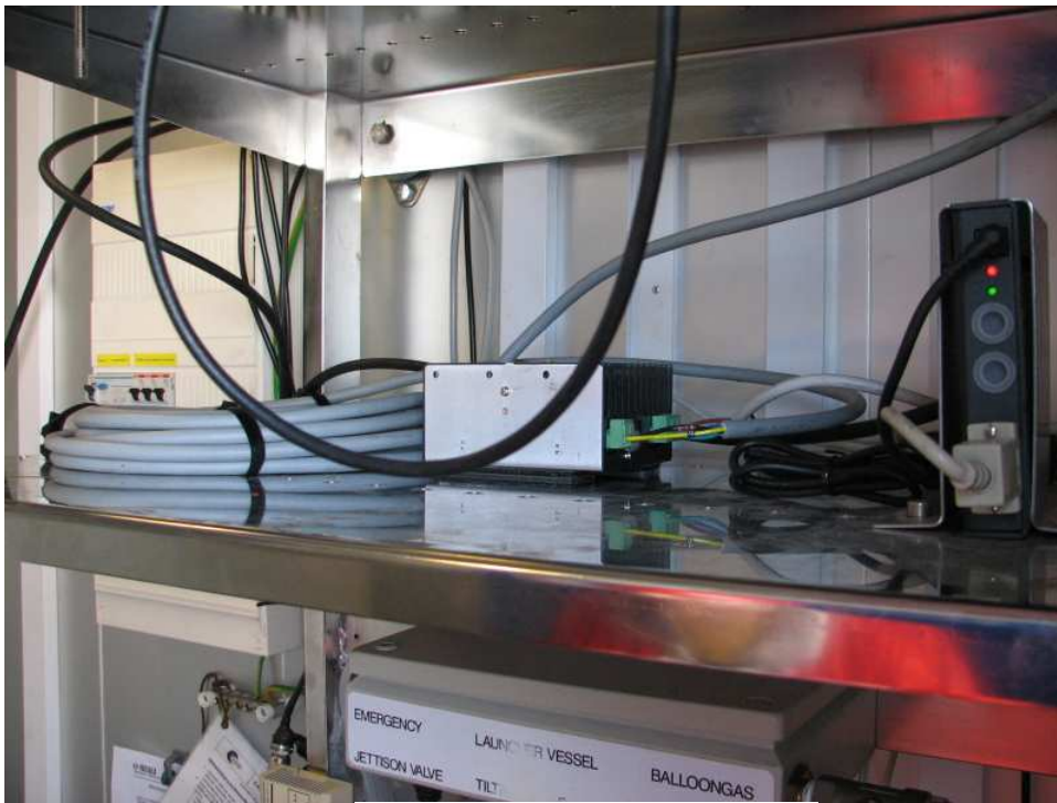
fig.6 – TRACO powered in a tight area
