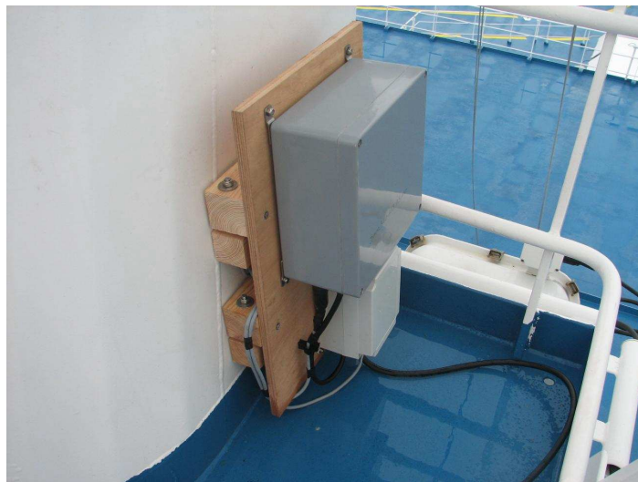
fig. 5 - BaRos fixed vertically on a mast
