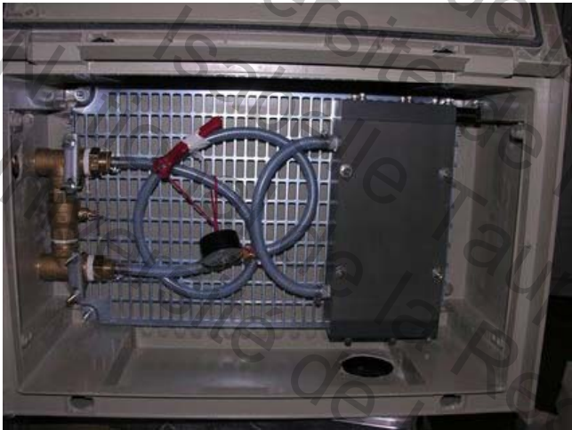
SBE45 bypassed for tests
